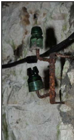
Glass insulators on the tunnel wall.
