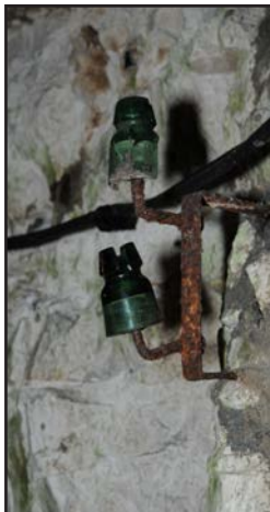
Glass insulators on the tunnel wall.
