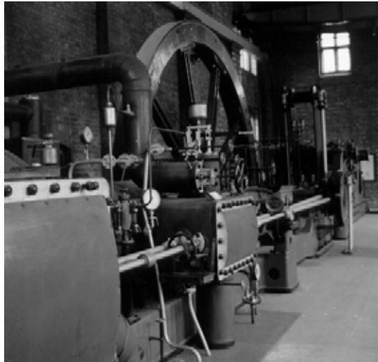
Brindley Bank Pumping Station © JS Waterfield
