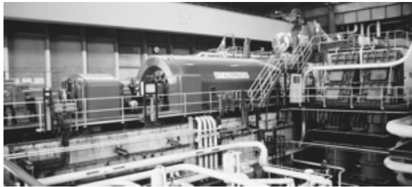
Gas Turbines at Rugeley Power Station
